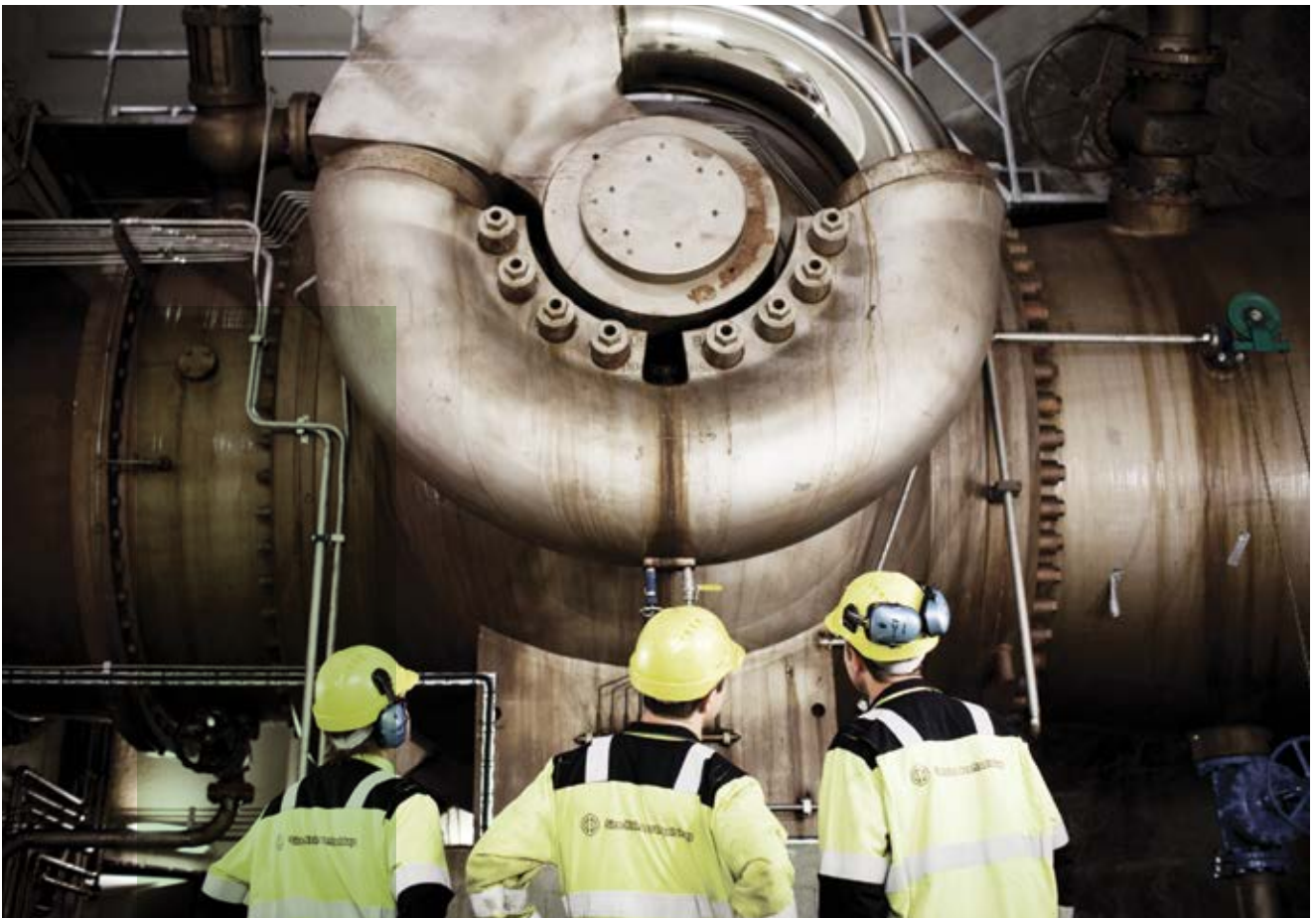
Turbine at a Sira Kvina power station. Photo: Sira Kvina kraftselskap
